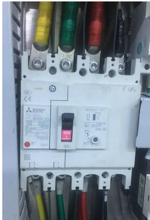
( Figure 5-2 Main air breaker )
