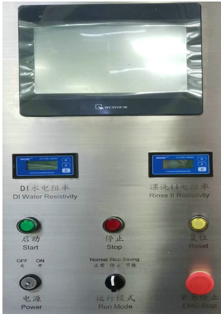
( Figure 5-1 Control panel)
